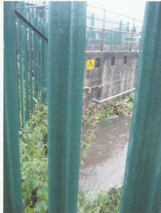
Debris at the outfall
